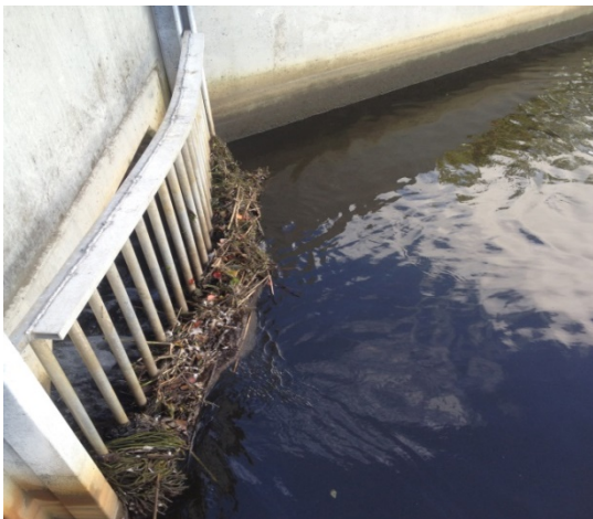
Figure 3. Wrack collecting on grates on the upstream side of the new culvert under Stewarts Creek during ebb flow.
